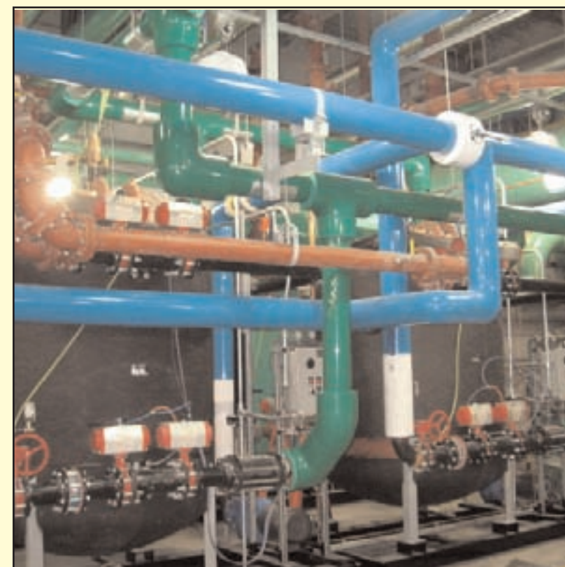
Condenser and Chilled Water Piping and Sand Filtration Tanks
