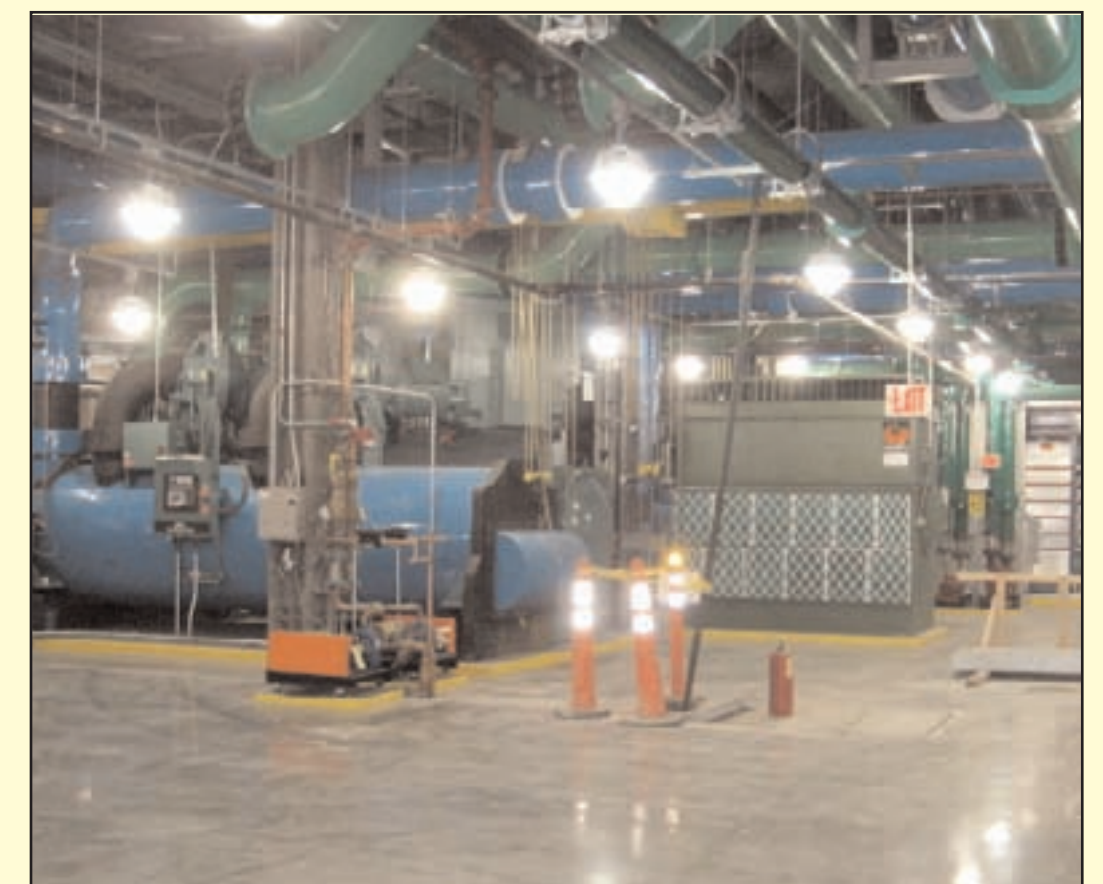
B4 Level Chiller Plant w Chiller and Air Rotation Unit
